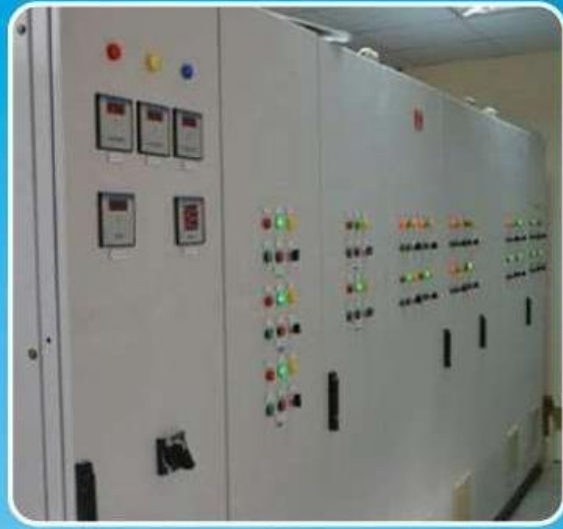
SCADA Controlled MCC Panel for Chemical Plant
