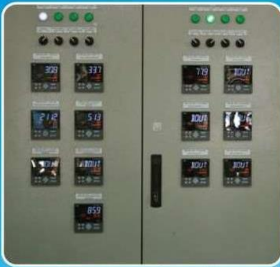
Heat Control Panel For Chemical Reactors
